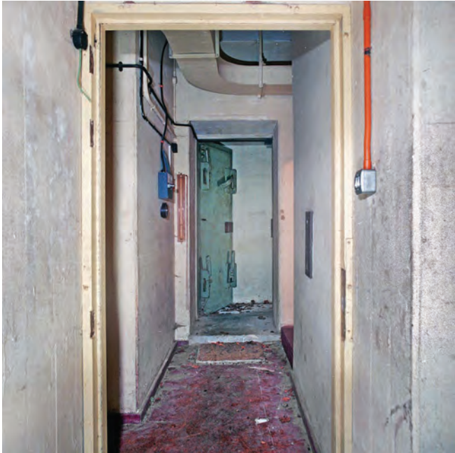
The impressive-looking blast doors with secure catch. This was the entrance in use in the old building, just inside the dog-leg corridor (to minimise blast pressure). Photo Nick Catford
